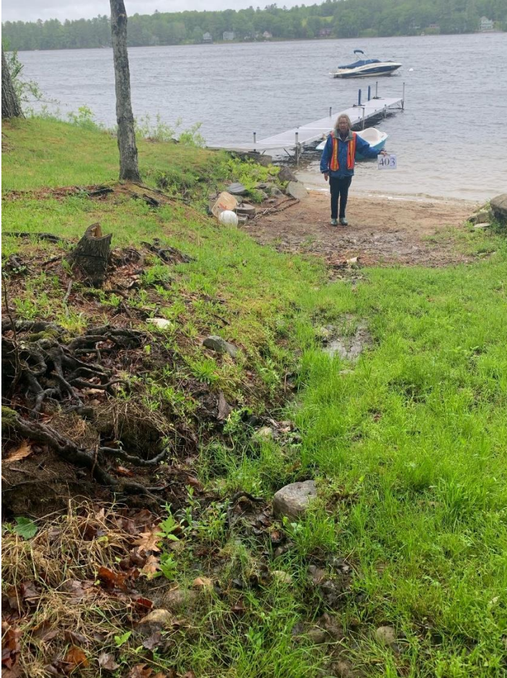
Figure 21: High Impact Private Road Site Rill/Gully Erosion leading directly to lake.
