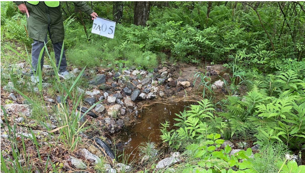
Figure 22: High Impact Town Road Road shoulder erosion and sediment deposition directly into stream
