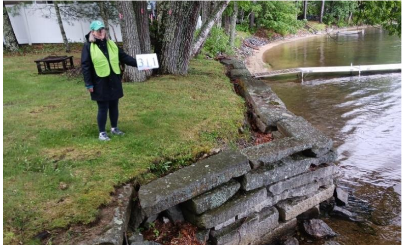
Figure 9: More dramatic erosion identified on a residential site.
